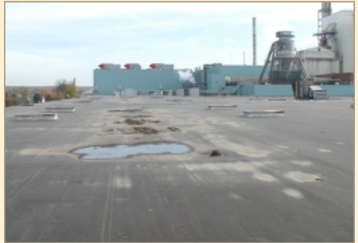
It had been over a week since the last rainfall when this picture was taken. The years of ponding water and accompanying debris accumulated on the Hyload membrane has not caused any damage.
