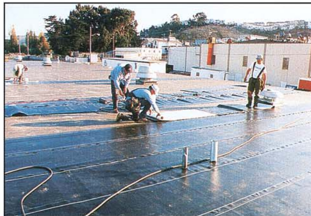
CTEM weathering membrane is installed on top of the CTEM base sheet.
