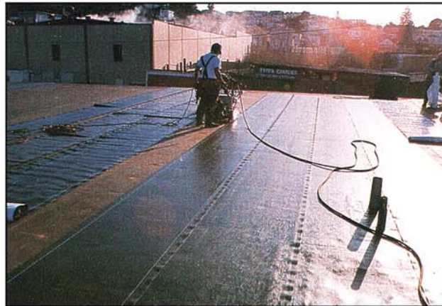
All CTEM laps and termination points of the weathering membrane are hot air welded.
