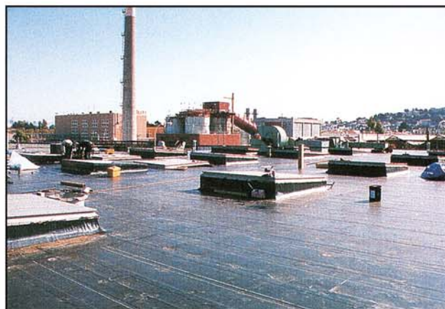
Completed CTEM roof is in excess of 125 mils of total CTEM products.
